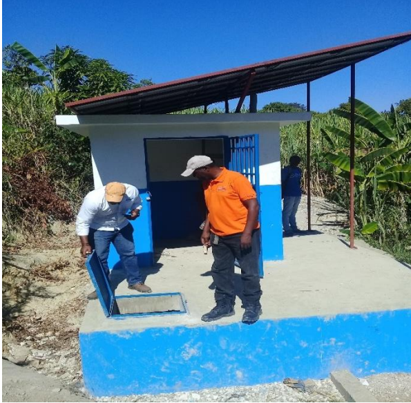
Grand Boucan – Water system with solar pump
